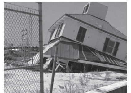
A toppled Coast Guard tower. Photo courtesy of April Halprin Wayland.
